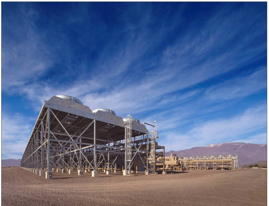
Enel's Stillwater geothermal power plant, Churchill County, Nevada. Photo courtesy Enel North America.
