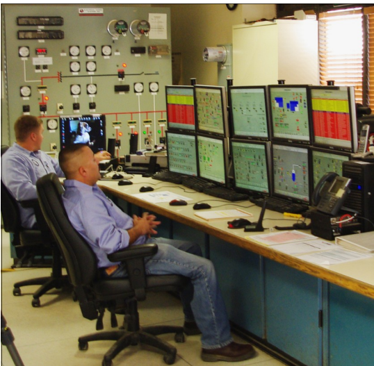
Local employees at a CalEnergy US geothermal facility in Imperial Valley, California
